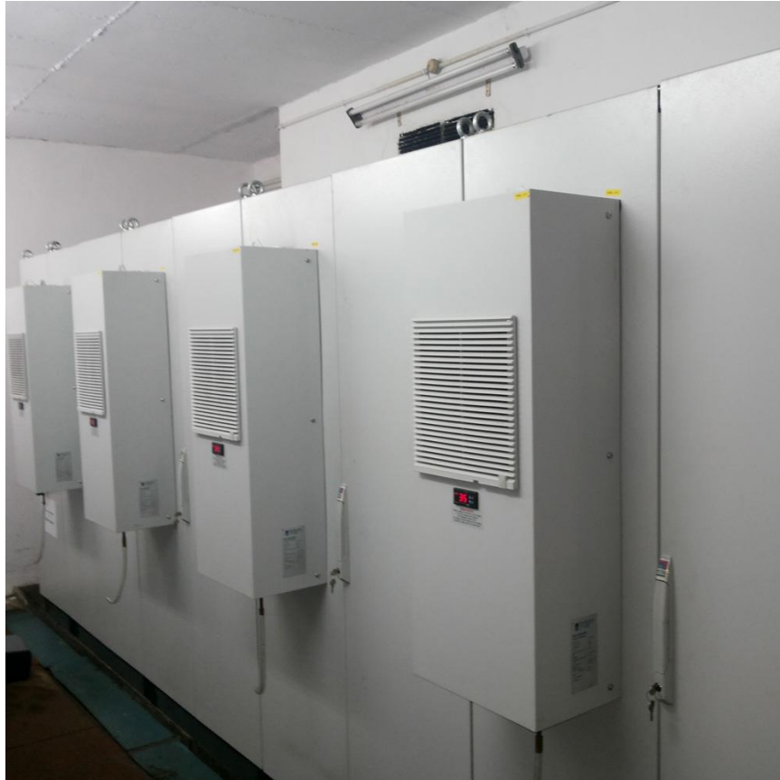
airconditioned electric cabinet
